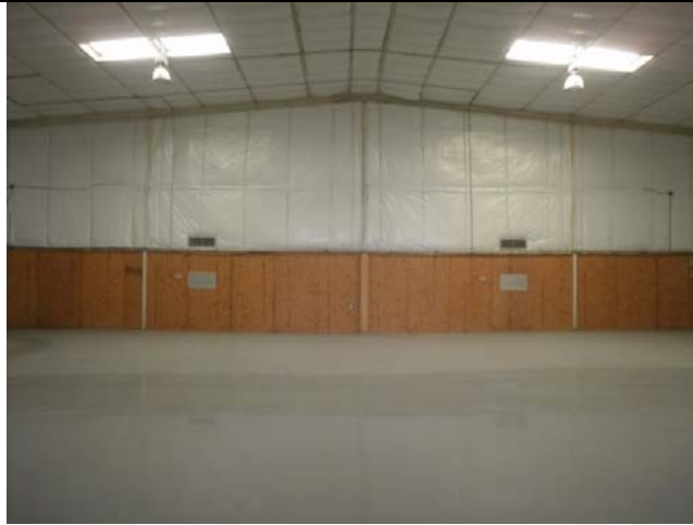
New layer of vinyl faced insulation, epoxy floor coating & A/C wall package units
